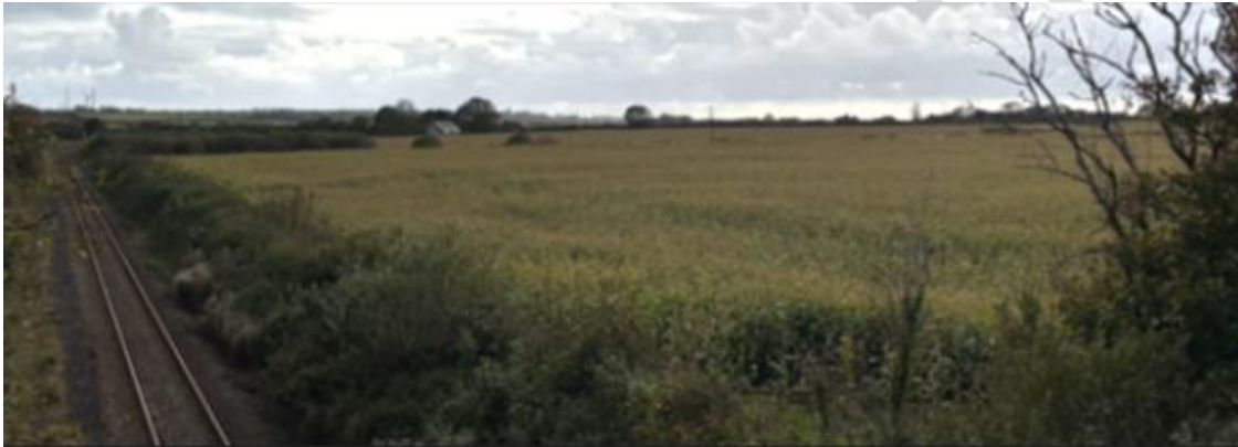
Photo 12: Mixed Subgrade 3b and Grade 4
