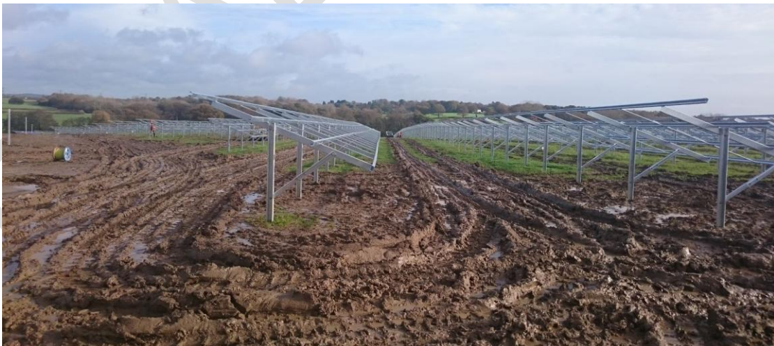
Insert 12: Panels Installed in Poorer Conditions
