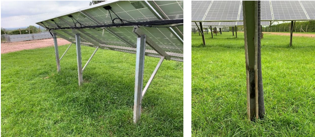
Inserts 15 and 16: Cabling along Panels (Manor Farm, Llanvapley)
